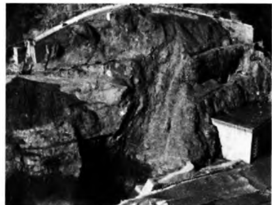
Photo 6: View of right abutment showing slide scars and effects on tail track
