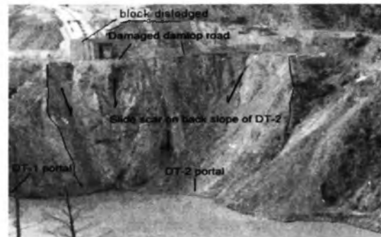
Photo-3: Right bank - Back slope of DT inlet portals with multiple slides
