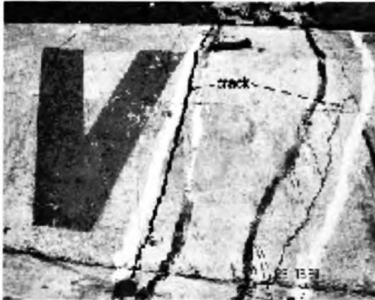
Photo-4: Transverse cracks in the tail-track
