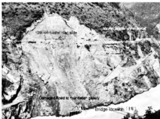
Photo-2: Damages to roads left bank
